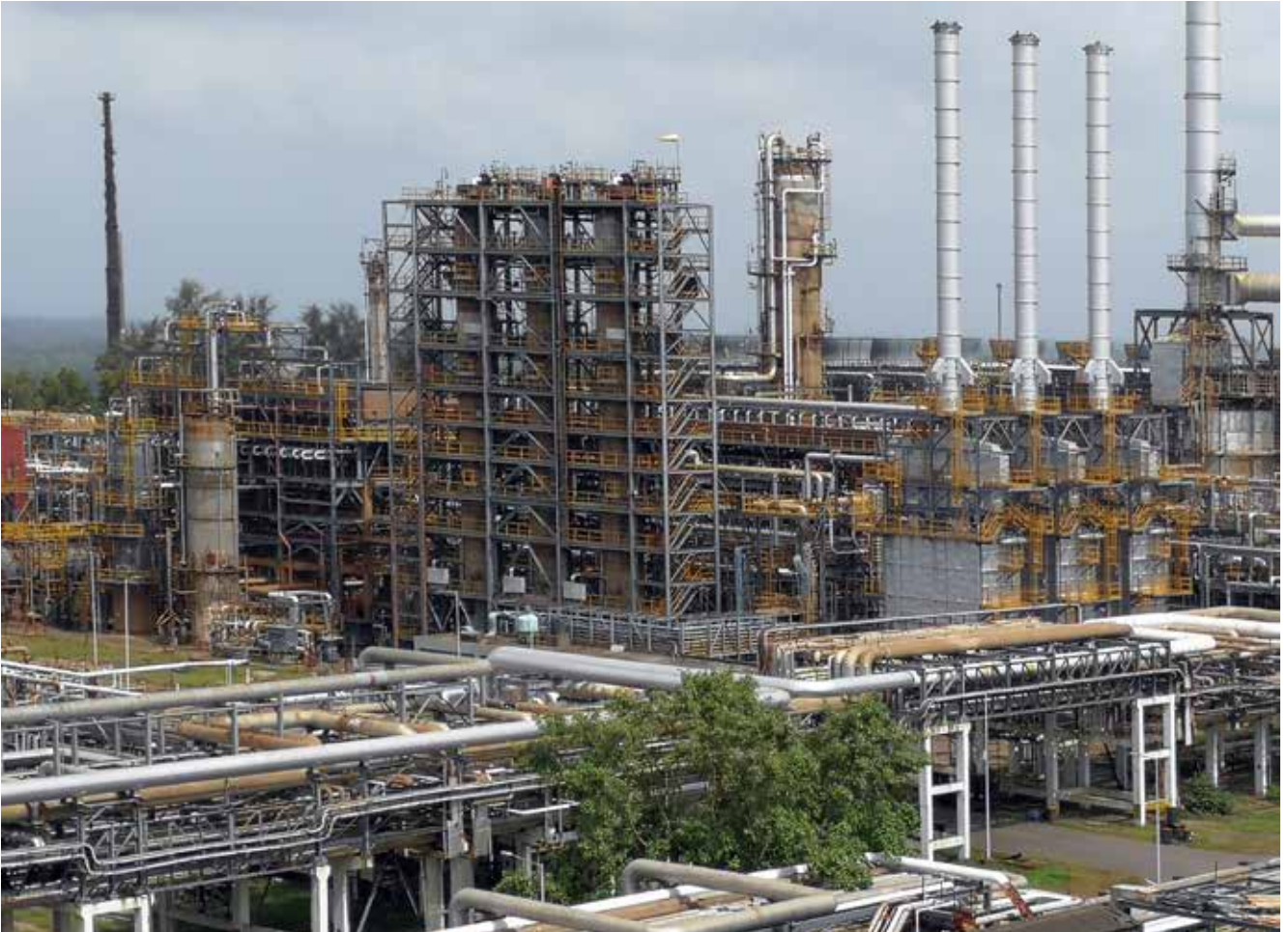
Mangalore Refinery Hydrocracking Unit no. 1
